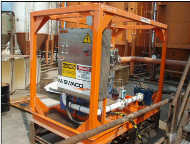
Figure 1. High-shear mixing unit installed on LMP.
