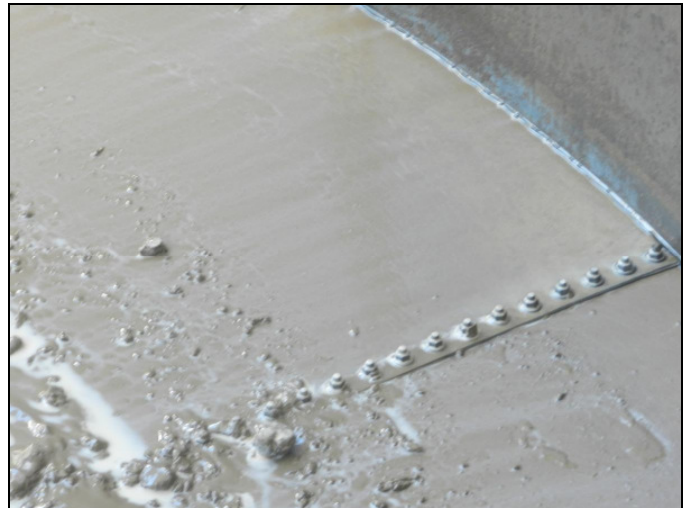
Figure 11: Inside the tank is considerably cleaner with solids easily dispersed in water.
