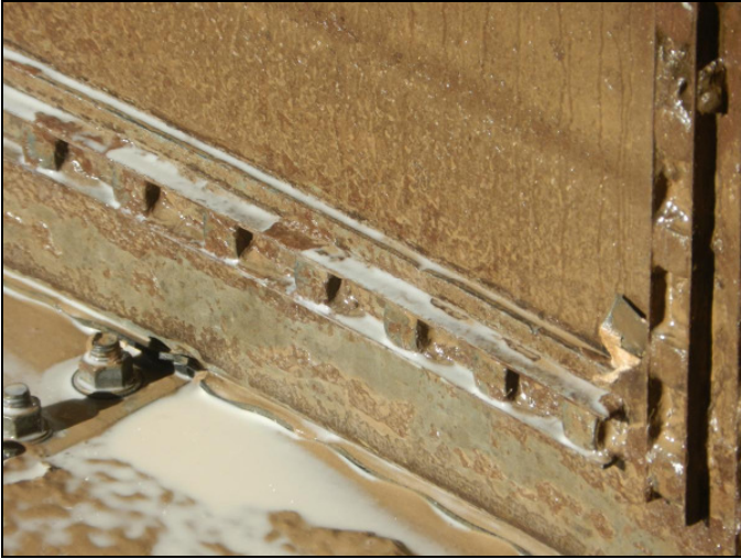
Figure 12: Sides inside the mixing tank where there was maximum agitation were completely free from oil-wet sediments.
