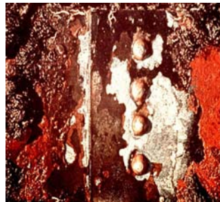
Figure 6 Galvanic Corrosion from low velocity seawater
