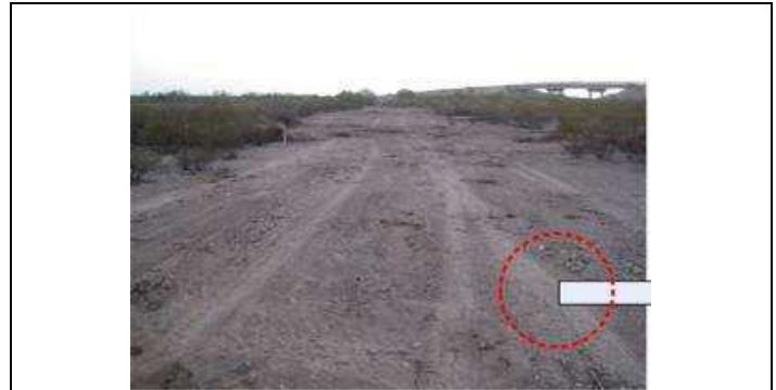
Figure 3 represents a site view ready for road construction. The area was cleared with a brush hog, but not graded. The entrance ramp to the test facility is shown in the background.
