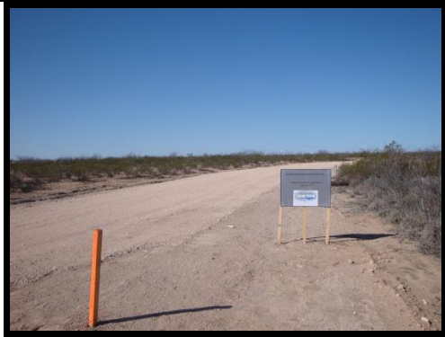
Figure 5 shows the completed SESI road. The segment of the road was laid out in such manner as to join the two other types of road and offer an alternate route to the offices to the staff at the test center.
