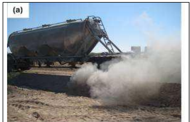
Figure 3a shows the road material being placed on the prepared base. The entire construction of the road required less than 8 hours.
