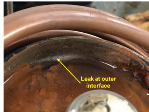
FIGURE 19 SMALL SCALE OUTER FAILURE
