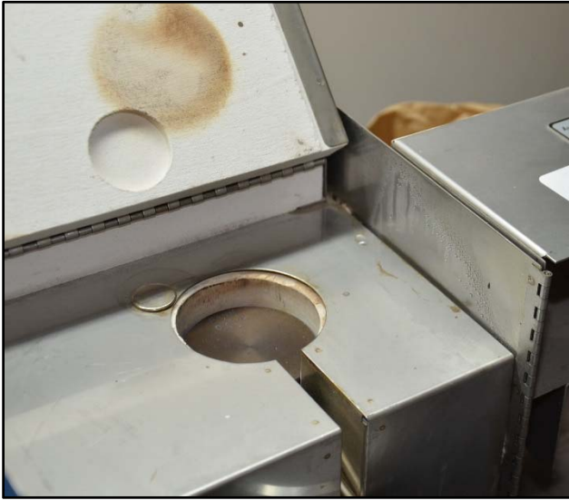
Figure 1: Condensation build up inside Housing
