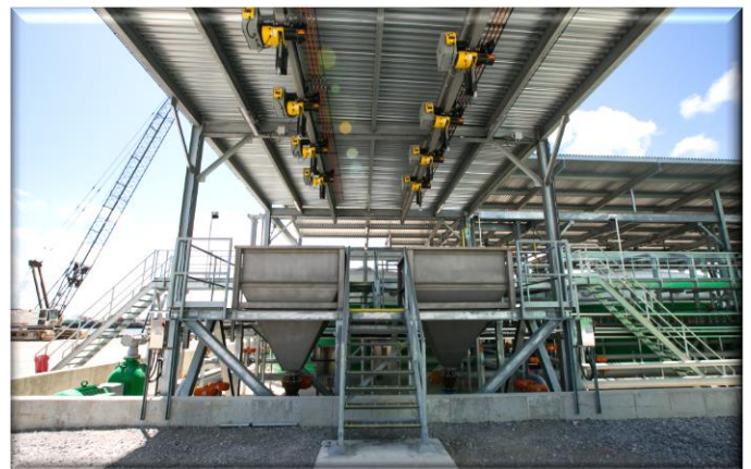
Figure 7 – Bulk salt delivery system
