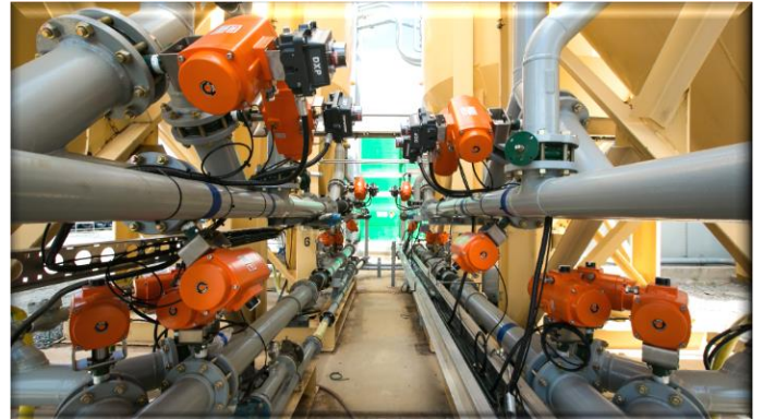
Figure 6 – Automated control valves
