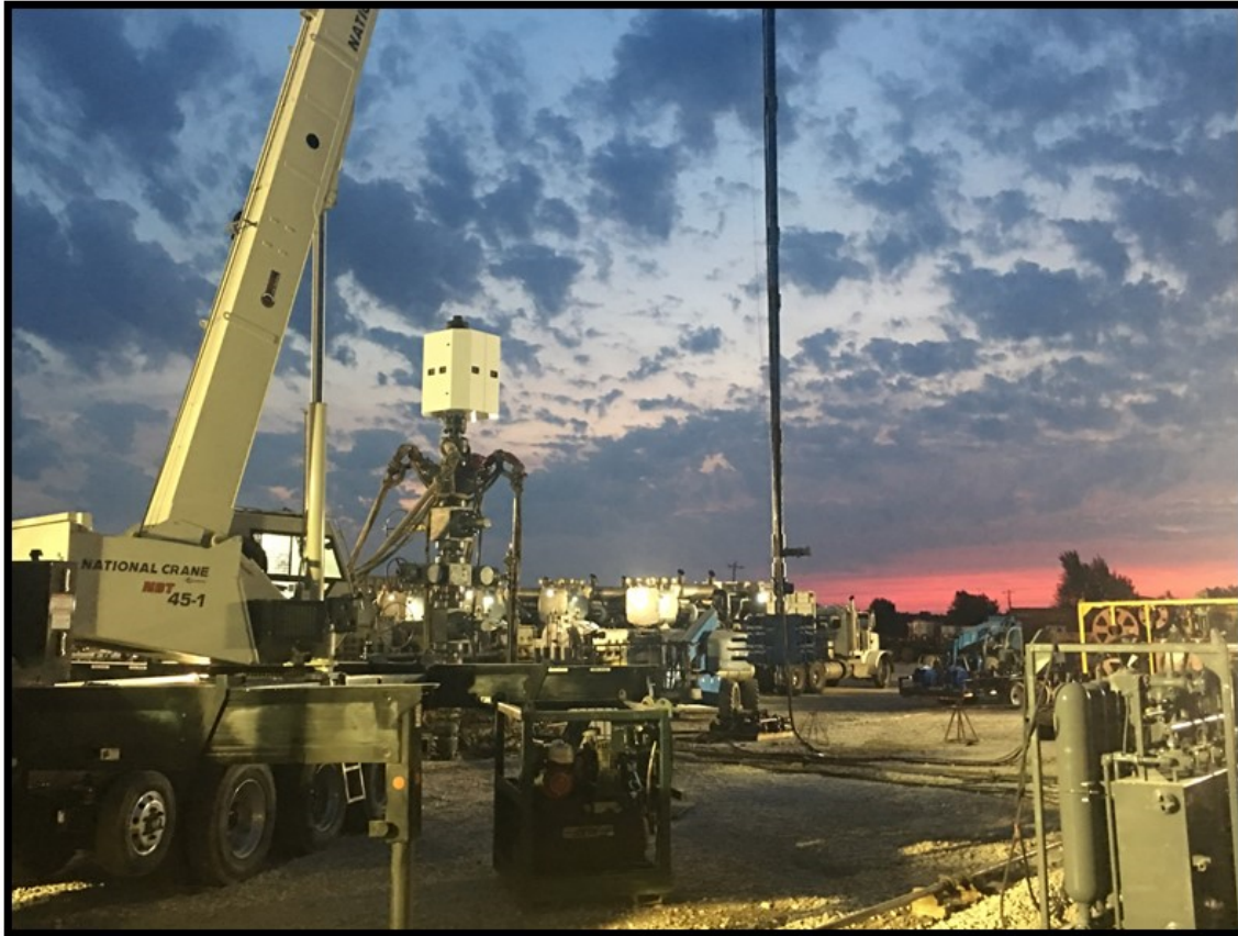
Figure 7. Multi-chamber Valve on Location in Oklahoma
