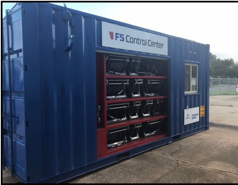
Figure 3. Control Center Enables Remote Actuation of Valve and Latch
