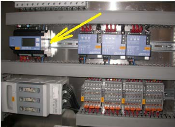
Fig 43 : Example of physical size of remote PQ monitoring system
