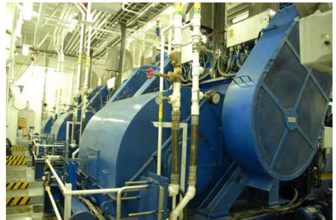
Fig 1 : Mud pumps controlled by adjustable speed drives
