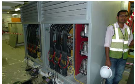
Fig 15 : 2 x 2300HP/1800kW D type wide spectrum filters on mud pumps during ABS compliance testing in the UAE
