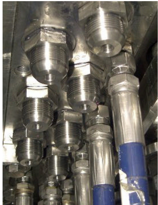
Fig. 27 - Flow restrictors as installed on a rig
