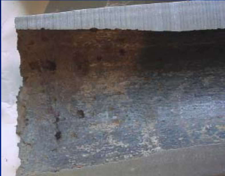
ID Corrosion pitting.
