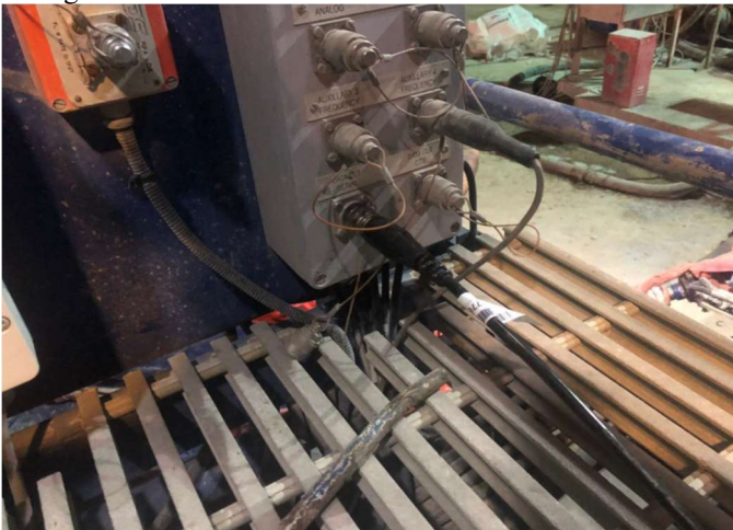
Figure 19: Ethernet Data Cable Connected to Cement Pumping Unit Junction Acquisition Box
