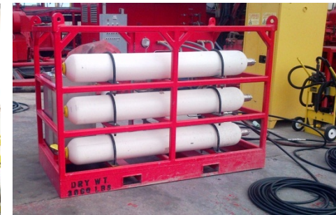
HPU to operate hydraulic motors
