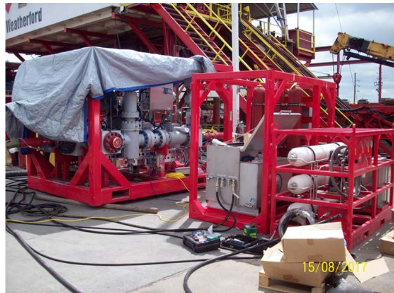
Mud flow control Manifold
