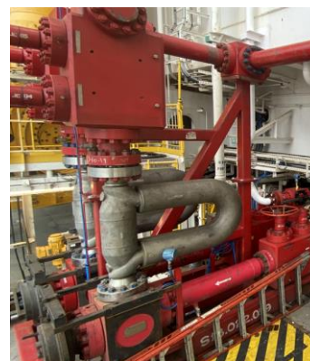
Figure 1: Coriolis meter installation on a drilling rig.
