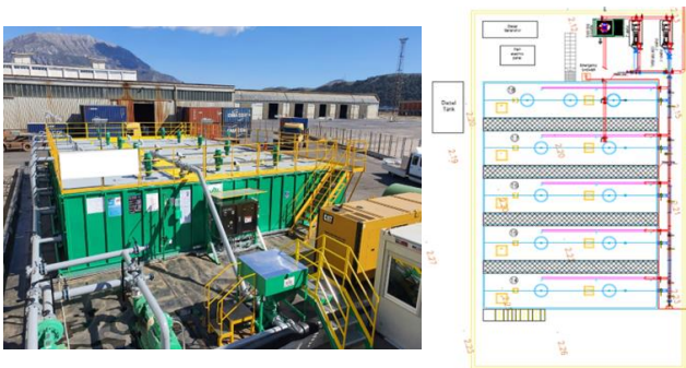
Figure 8: LMP for storing and mixing fluids at the supply base
