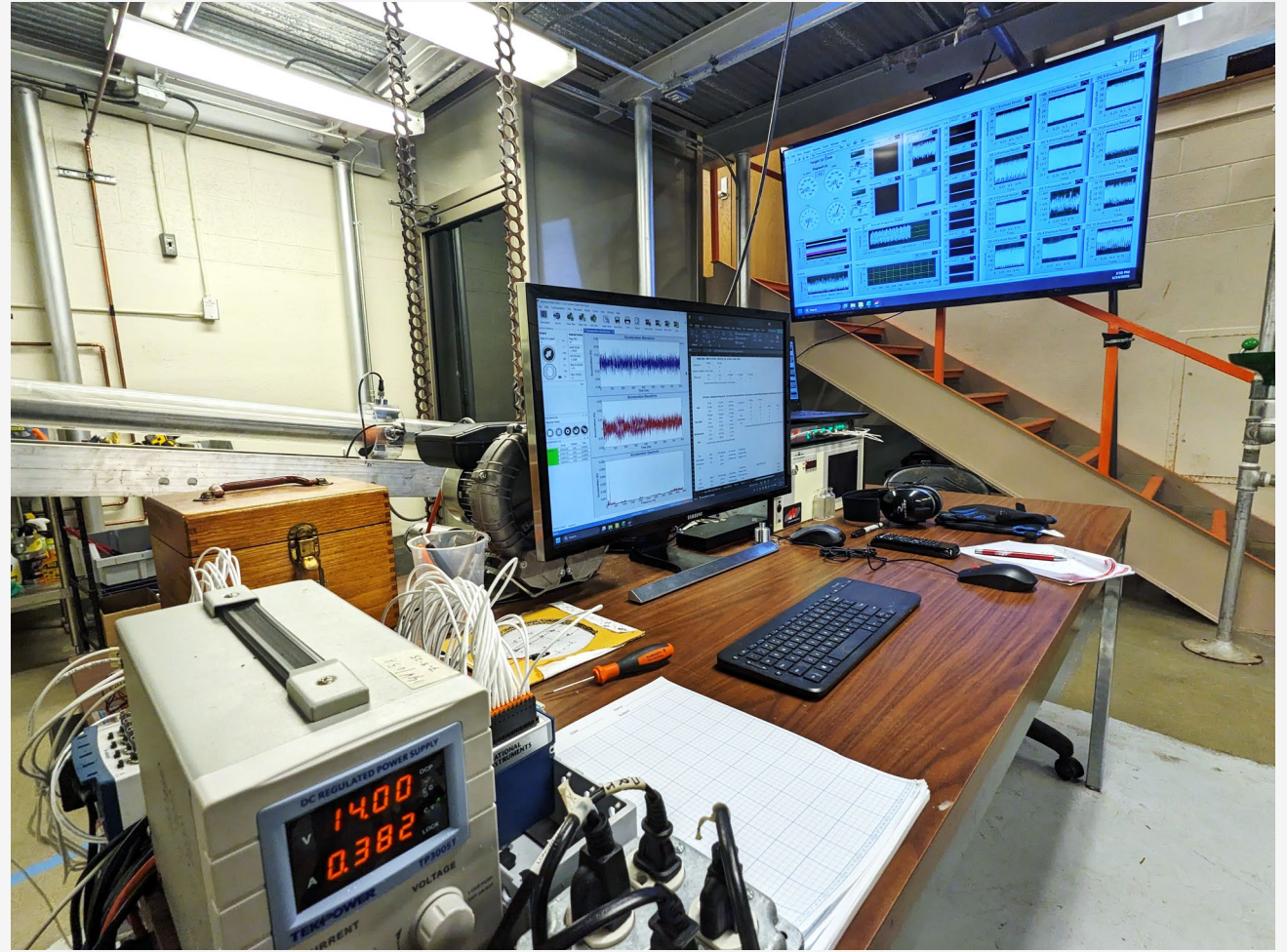
One Central Control & Monitoring System
